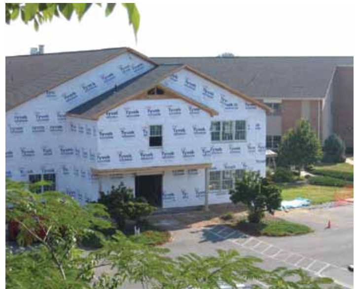
By late July, the installation of windows and insulation had been completed in the Birch/Fir addition.
