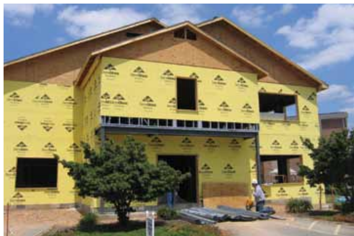
Expansion of the Birch/Fir wing began in early May with the construction of this two-story addition. With the exterior shell completed, most of the work has now moved inside.
